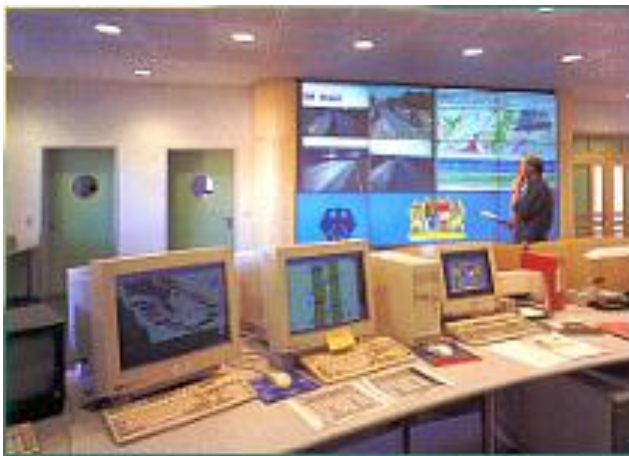
Figure 7-11 Typical Control Centre
